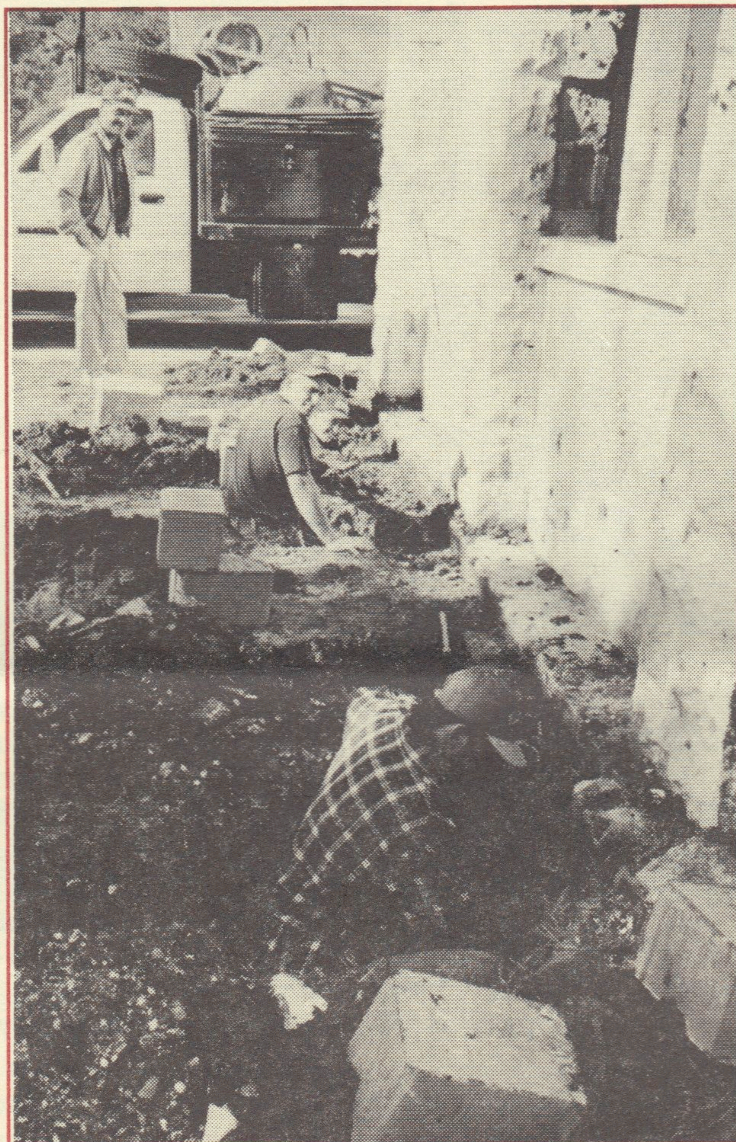
A crew works below the rear of the old St. Martinville city hall to shore up the nearly 100 year old building that is being renovated to serve as the Acadian Memorial. Work was begun with a "bricks and mortar" award of $15,000 from the Governor's Office of Rural Development sponsored by State Representative Sydney Mae Durand. This was followed by capital outlay of $75,000 for the project by the City of St. Martinville. (Teche News Photo)
