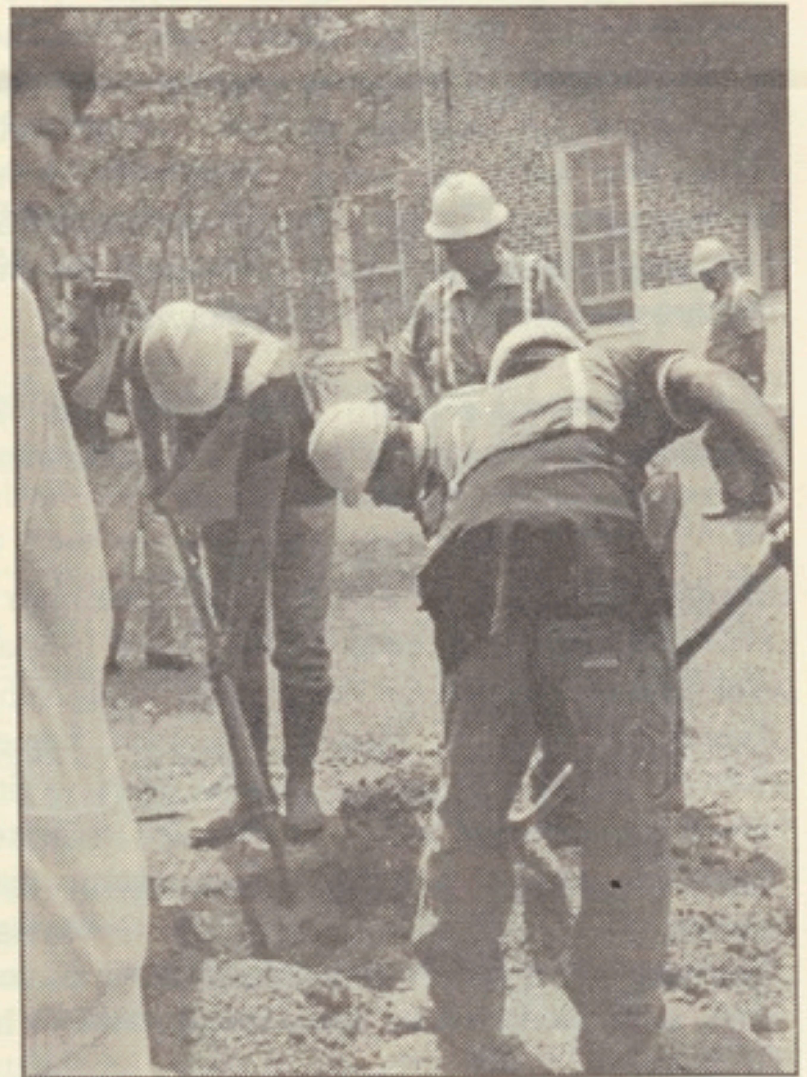
Above: City of St. Martinville employees excavate the time capsule in Evangeline Oak Park as onlookers anxiously wait
